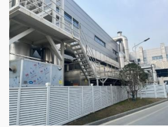
Exhaust gas treatment device
