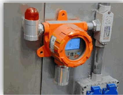
▶ Intelligent explosion-proof control real-time monitoring system
