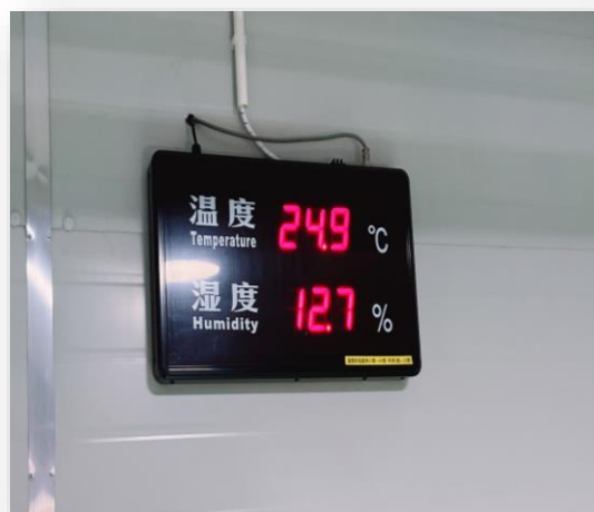
Intelligent temperature and humidity control
